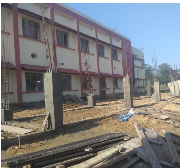
Jorhat Engineering College – Disabled Friendly Facilities
