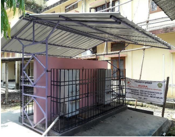
Drinking Water Facility at Abhayapuri College
