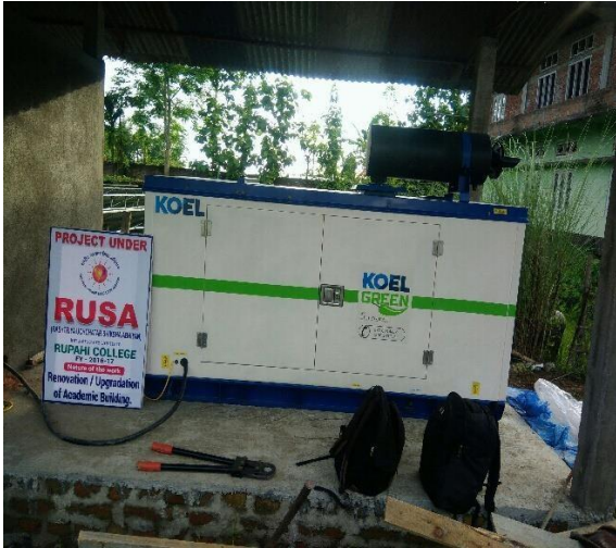
Purchase of Generator, Rupahi College
